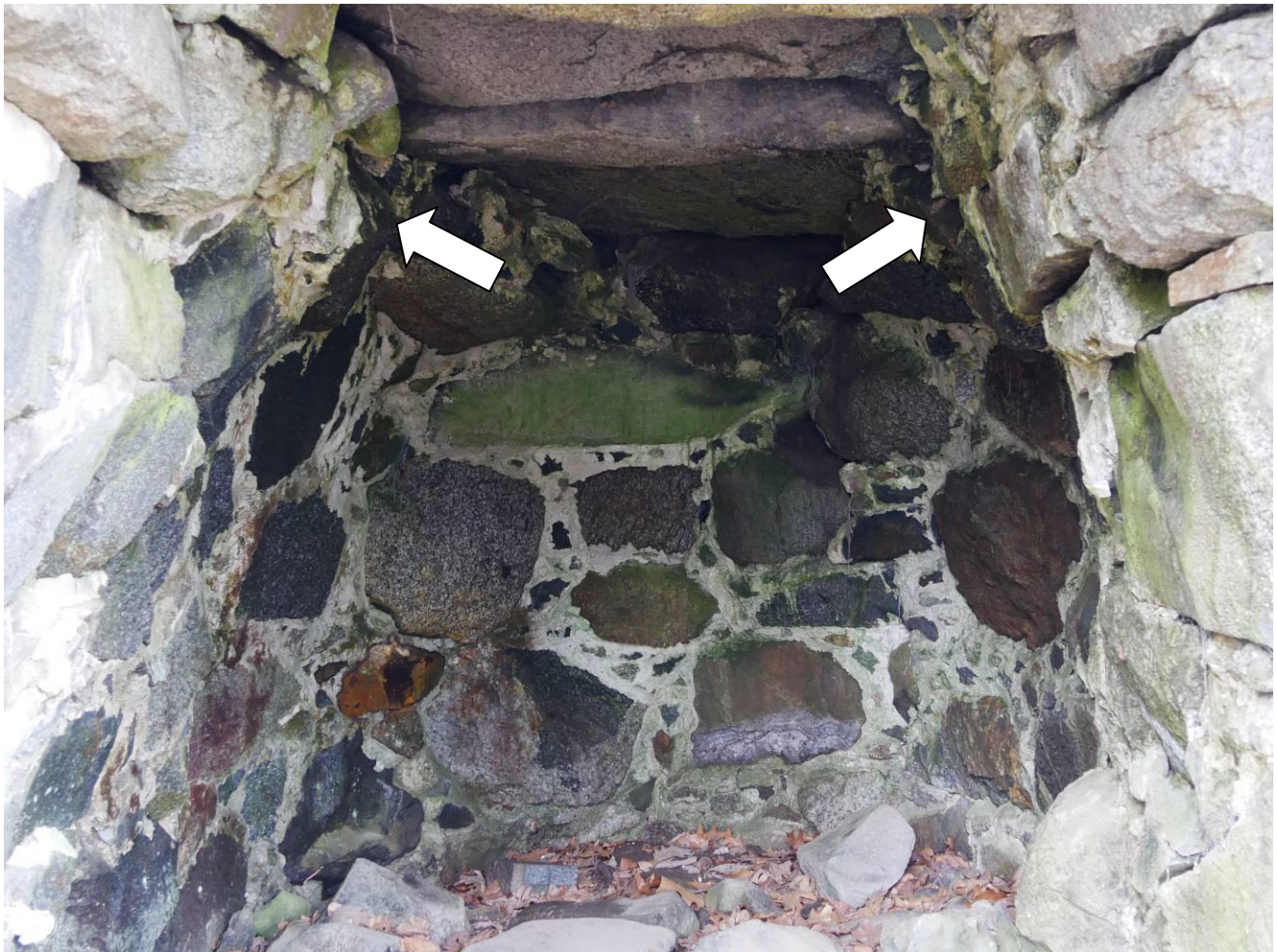
Figure 11 – Interior walls were pointed with mortar between 1920 and 1924 when it was used as a shrine to the Virgin Mary. Arrows indicate corbelling.
